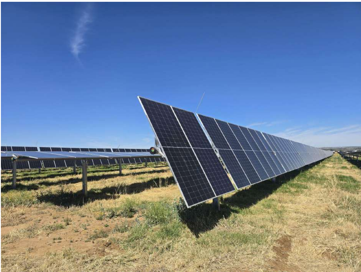
Tilted panels on site.
