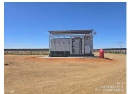
ITS in solar field.
