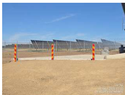
Conservancy tanks for O&M building.
