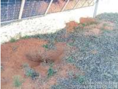
Positive evidence of faunal activity on site
