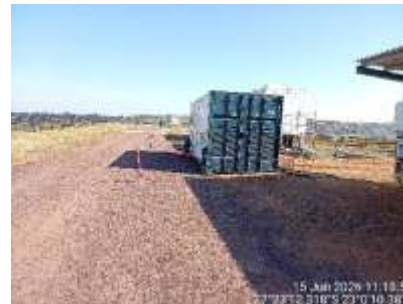
Temporary transformer in container with internalised bund.
