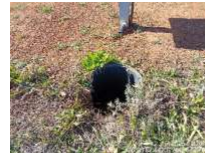
Infrastructure access point damaged.
