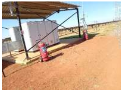
Fire fighting equipment on site.
