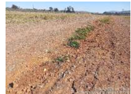
Internal road showing signs of erosion due to run-off.
