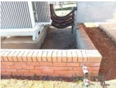
On site tranformer in adequately banded area.
