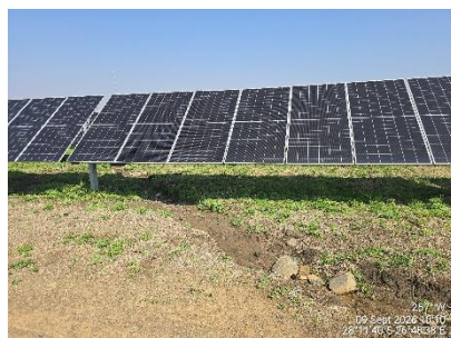
Erosion in solar facility to be repaired.
